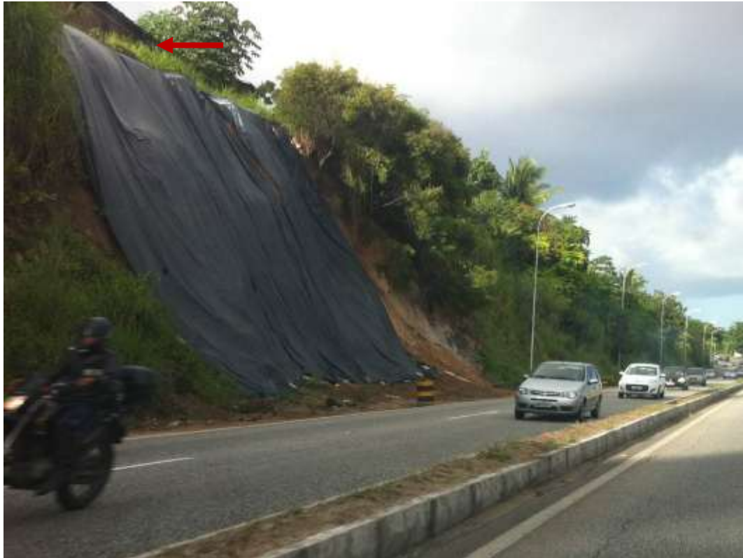
Figure 12: Landslide in João Pessoa City, BR 230 Km 19.
